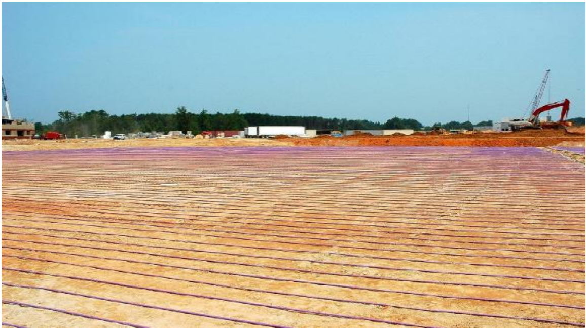
Purple Drip Wastewater Lines on Portion of Soccer Sports Field
